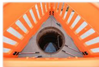
Protect Pedestrians From Work Zone Hazards
